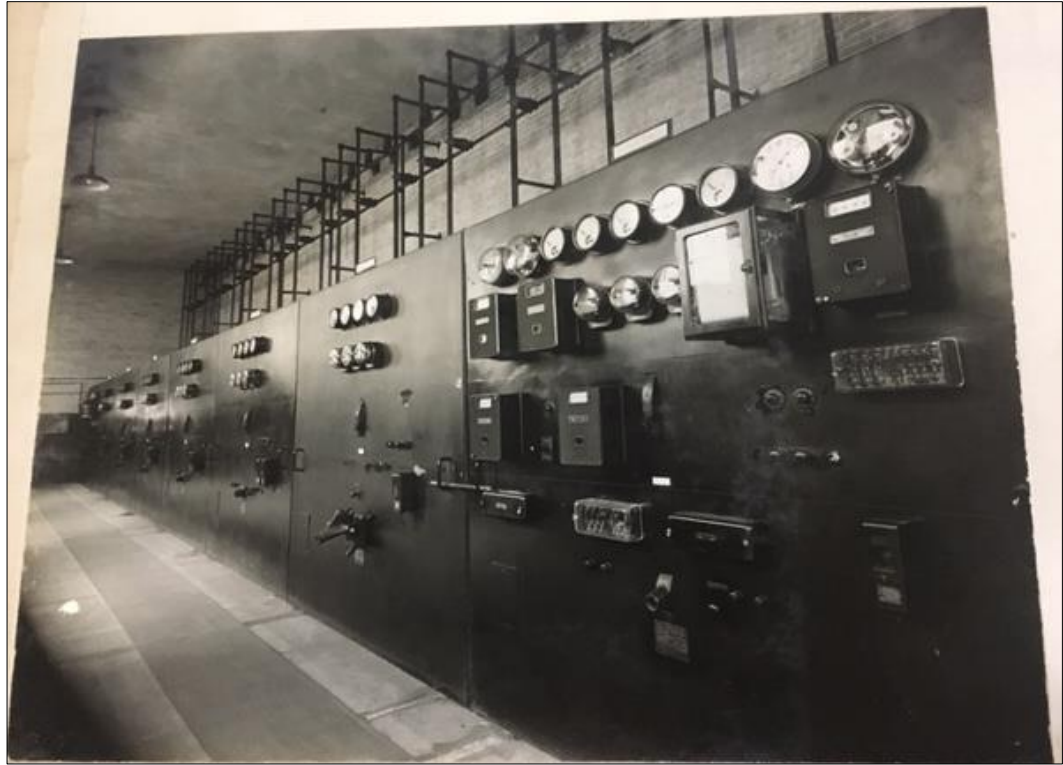
Figure 6: Interior of the Hauto Navigation Substation. The circuit breakers are on the north wall facing the Hauto Power Plant. The two incoming feeders are on the ends corresponding to the 11 kV single line.
