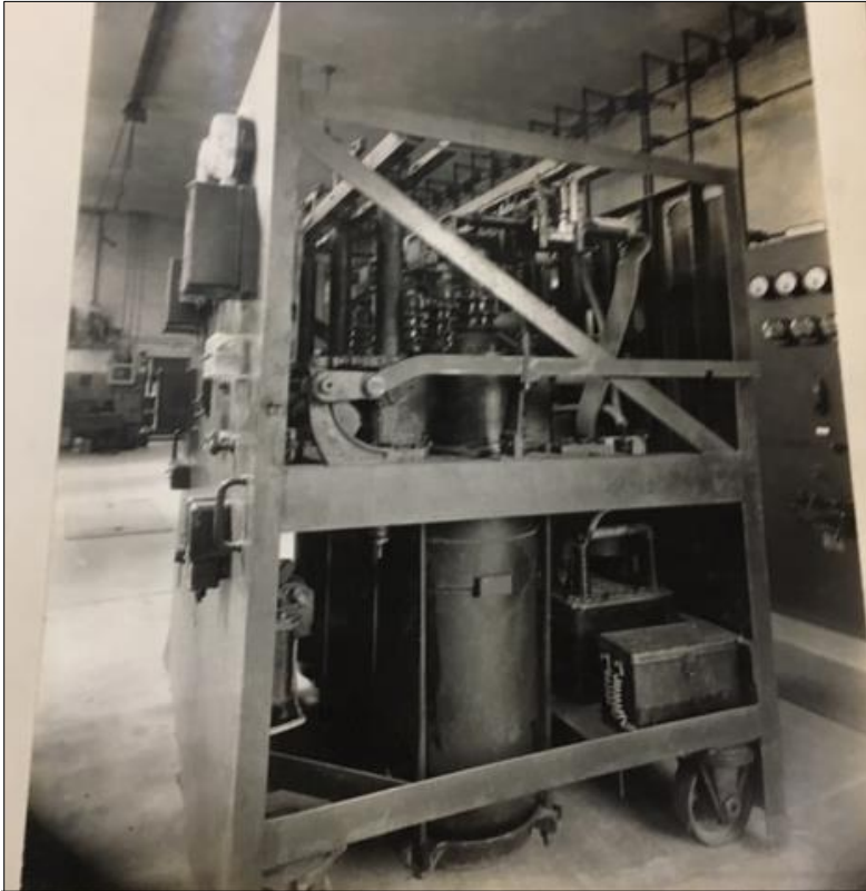
Figure 7: Hauto Navigation Substation draw out circuit breaker “truck”. There are three individual circuit breaker oil tanks in which the arc is interrupted. Only the first is visible because of the angle of the photo. Protective relays, projection mounted on the front of the slate panel, are part of the draw out circuit breaker assembly.
